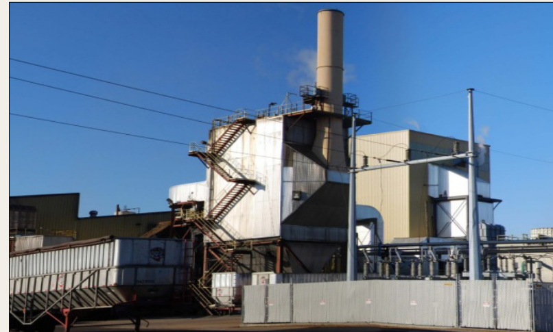
Controlled Energy Generation
